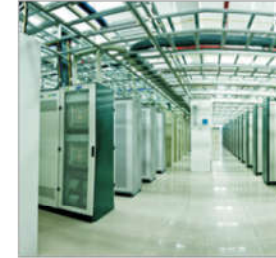
Mobile Data Center in Jilin Place: Jilin Area: 10400m 2 Panel Type: Calcium sulphate panel
